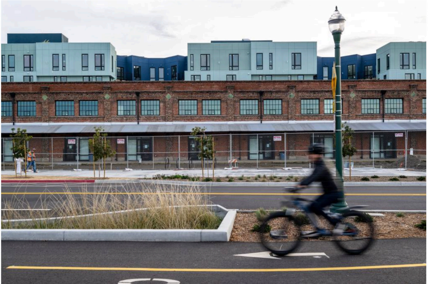
The Del Monte warehouse is under construction to become an apartment building in Alameda on Jan. 12, 2023. (Beth LaBerge/KQED)
